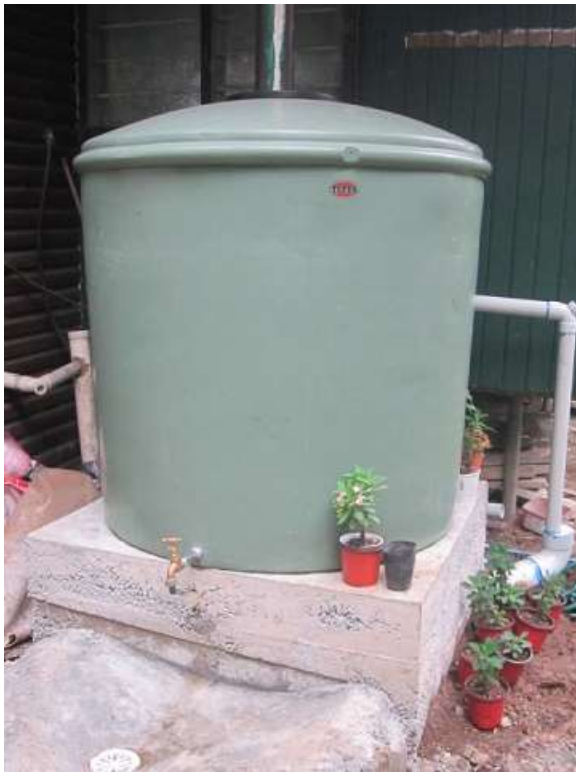
The newly installed water tank. The cement base is doubling as shelving for Miring's plants!
